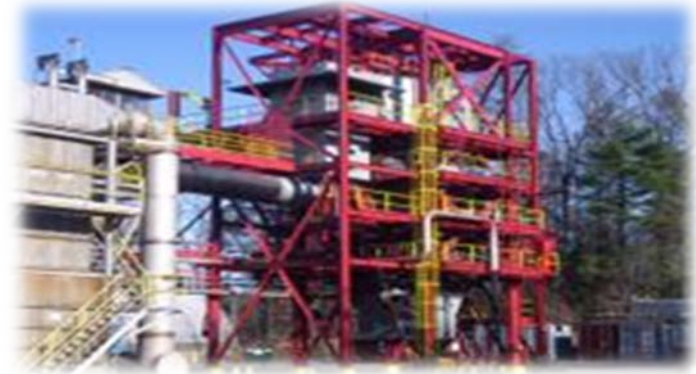
5 MWE Oxycombustion Pilot
